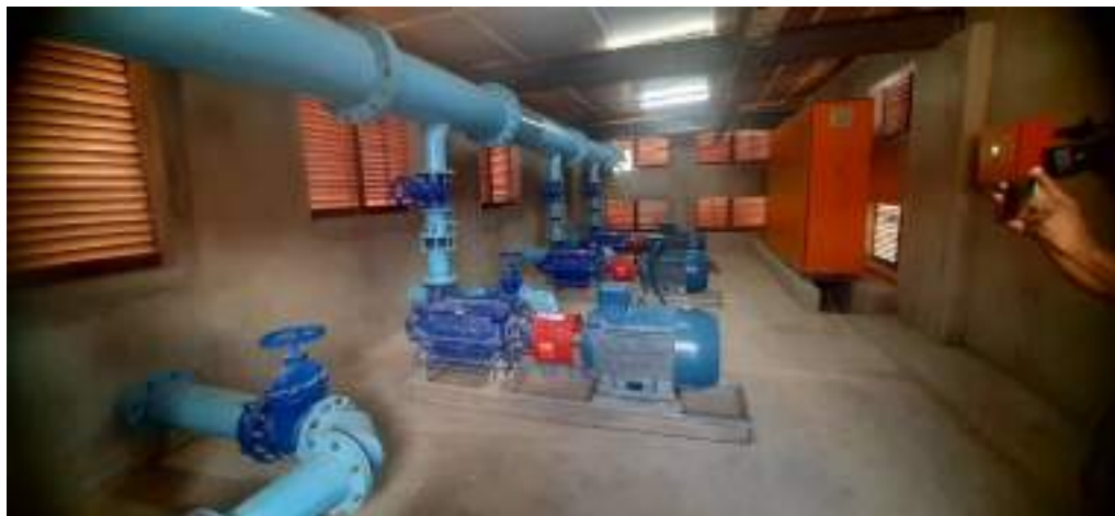
Water Treatment Plant at Chivhu dam
