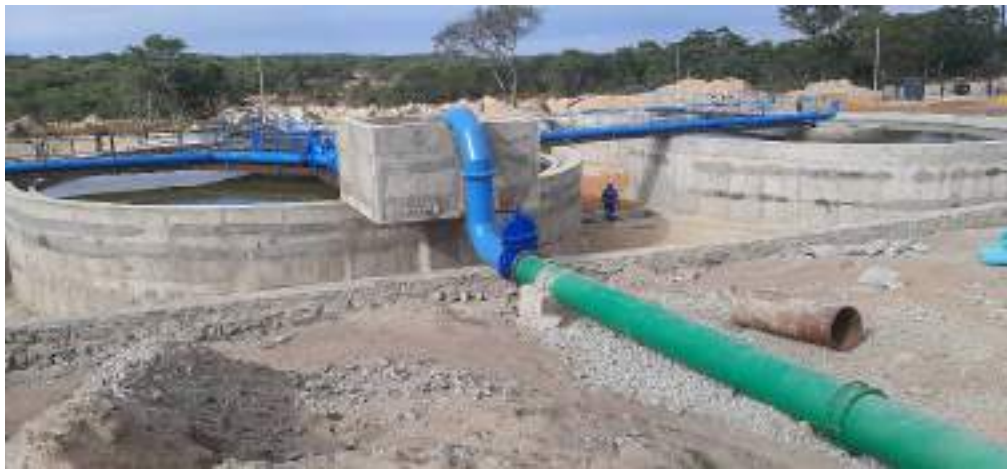
Water Treatment at Chivhu dam
