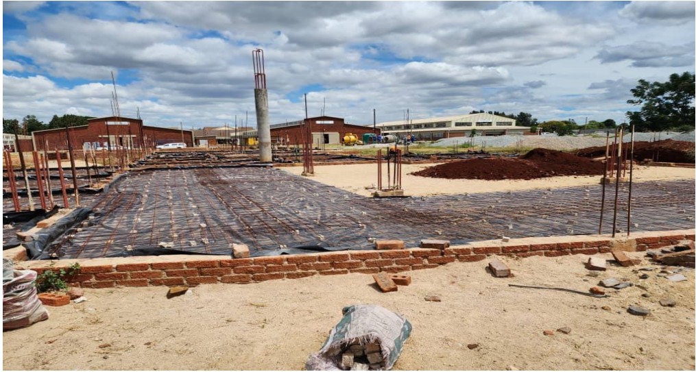
Substructure level of the southern side of the Multi Lab Plaza at Harare Institute of Technology
