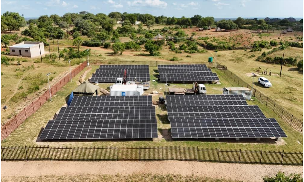
Hwakwata Community solar project in Chipinge
