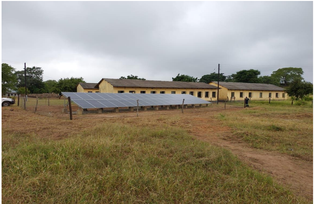
Mabhare Solar System in Masvingo
