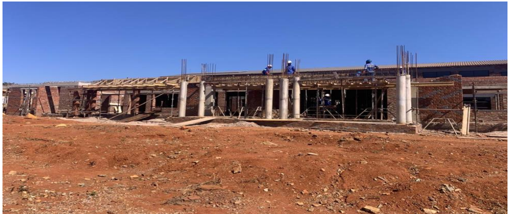
ZOU Administration, Teaching and Learning Block: Hatcliffe Campus Phase 1 Administration, Teaching & Learning Block Construction Project
