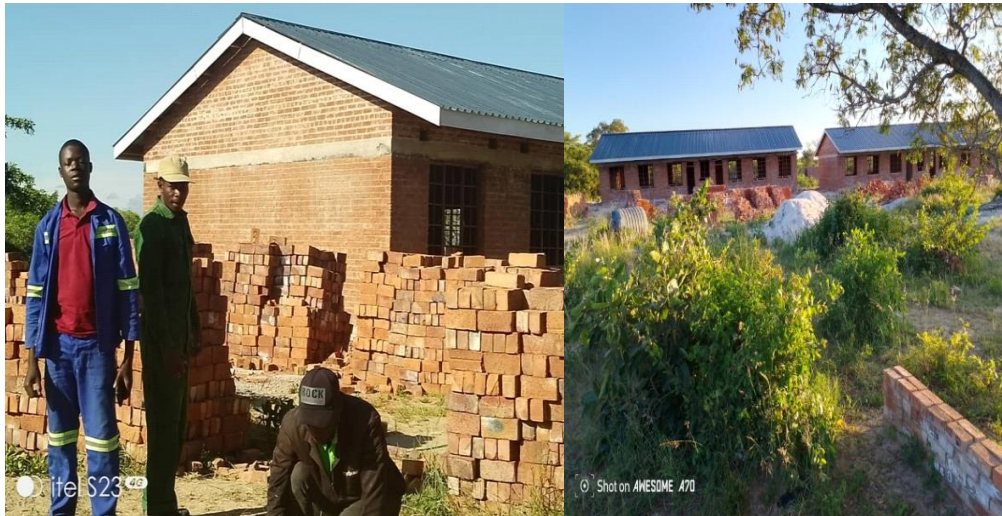
Mkoba Teachers Gangarabwe Practising School Phase 1: Gangarabwe High School Classroom Blocks being constructed by ISEOP Trainees
