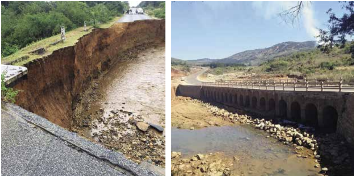
The Cyclone Idai Damaged Mvumvumvu Bridge in Manicaland was reconstructed during the First half of NDS 1
